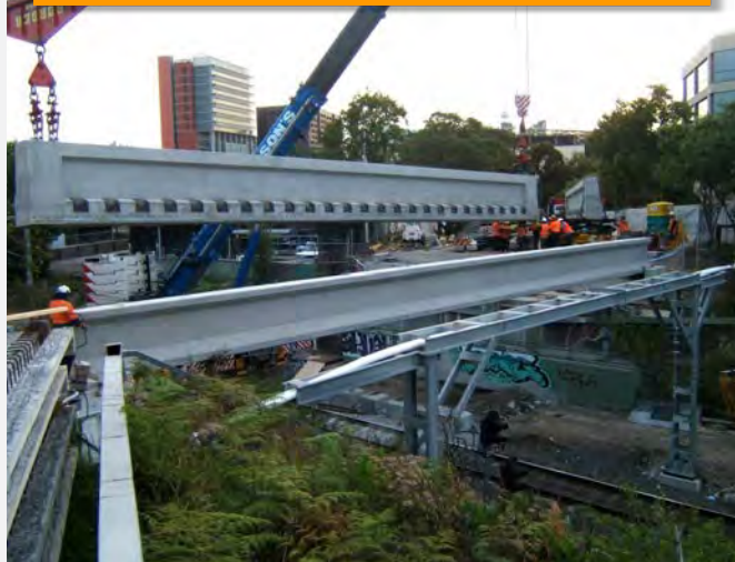
New Bridge for Old replacement at St Leonards, Sydney – Greg set out and monitored the placement of bridge abutments, bridge girders, each weighing 100 tonnes, and services – working blind until the old bridge was removed.
